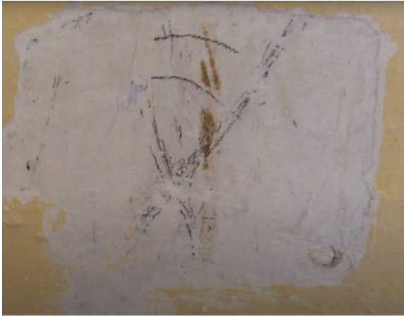
Figure 3. Cracks on the walls of Chalepas Museum revealing lines of sketches.
